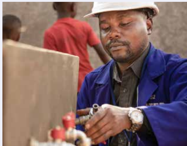
NWSC Staff installs a tap for one of the PSPs constructed in partnership with MTN during the Covid-19 Pandemic
