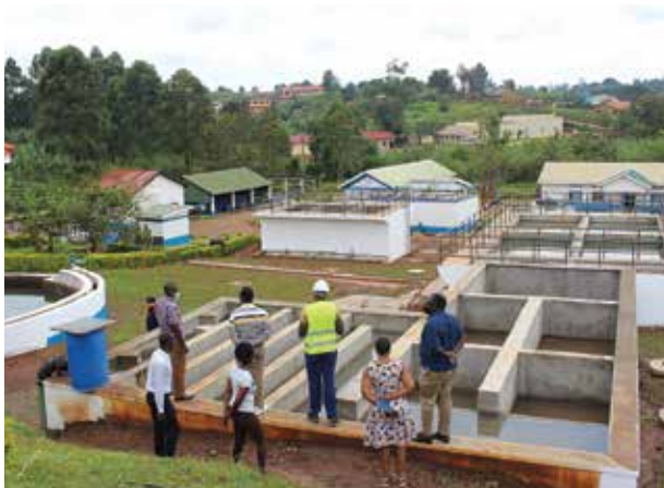
Upgraded Fort Portal Water Production Unit
